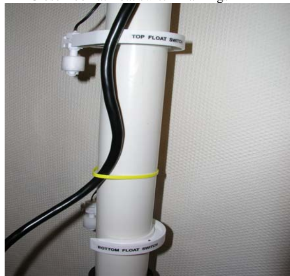
Closer look at float switch markings
